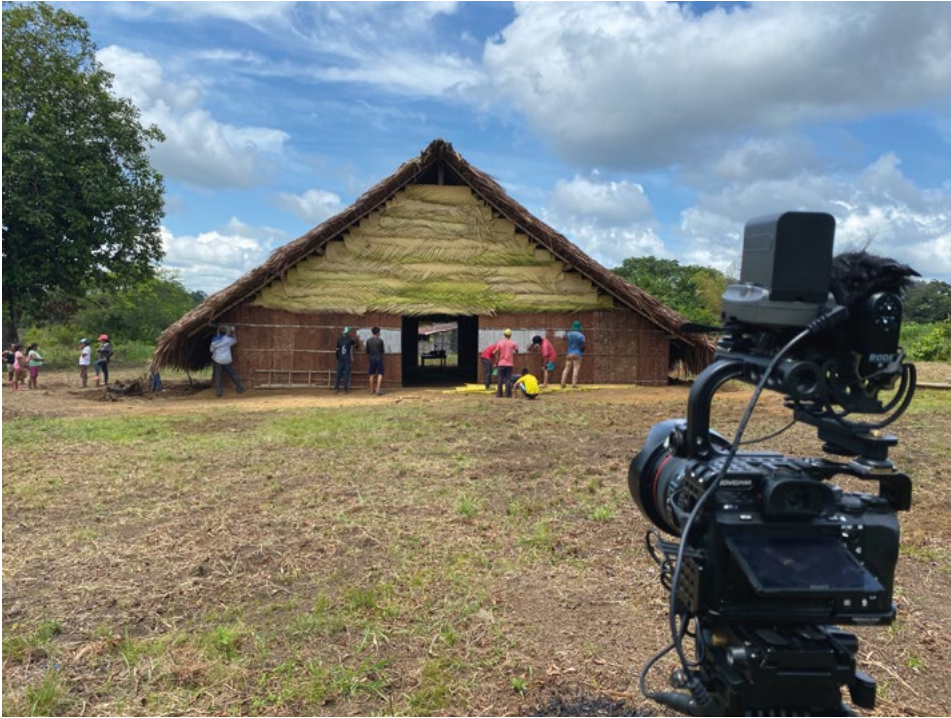
Fig. 1 Filming of the last step in the construction process. Photo: Mikko Gaestel, 2019
